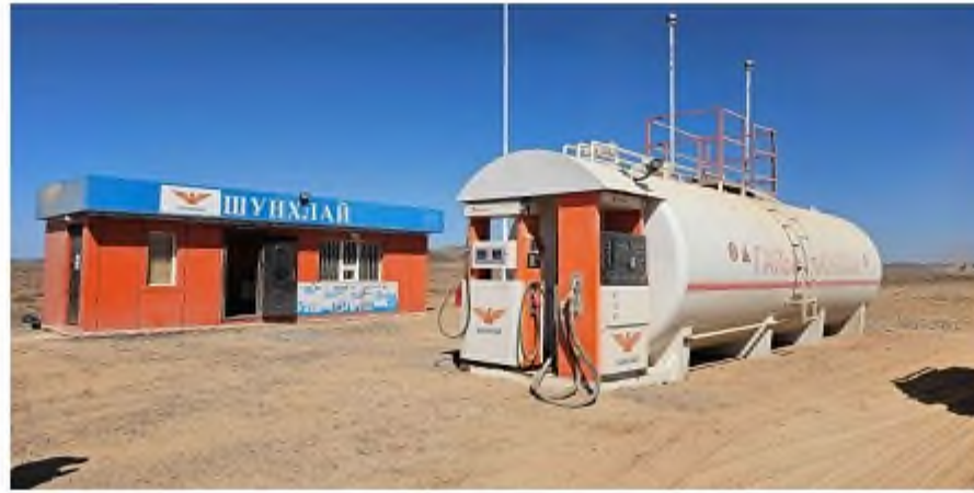
Temporary Fuel Station
