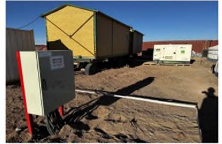
Ger Camp & Construction Power
